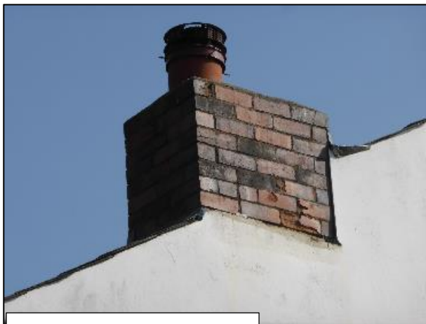
Poor render detail to South West chimney CH01
